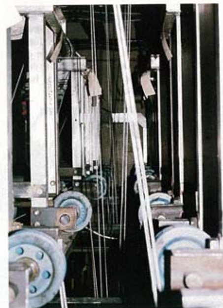
View on the fly floor between the double stacked rows of 23 winches.
